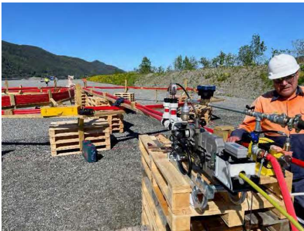
Figure 5. Installation of 18 mm cable in 40/30 mm PP duct, in total 2.54 km long, by floating
